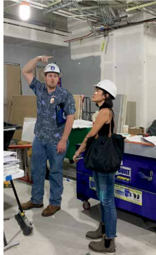
Catherine Kenjo, AHL associate project manager, discusses the existing conditions with Fred Morelli, project manager at J&J Worldwide Services, before the installation of a walk-in freezer at Tripler Army Medical Center—Nutrition Care Department. PHOTO COURTESY AHL
