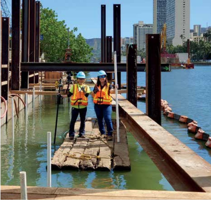
Hawaiian Dredging Construction Co. Inc. Project Engineer Marisa Yamada, left, and Cost Administrator Nani Blue work on the Ala Wai Canal Improvements project. PHOTO COURTESY HAWAIIAN DREDGING CONSTRUCTION CO.
