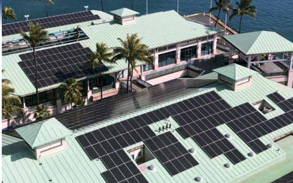
Holu Hou Energy designed Hawaii Pacific University’s Aloha Tower solar system.
