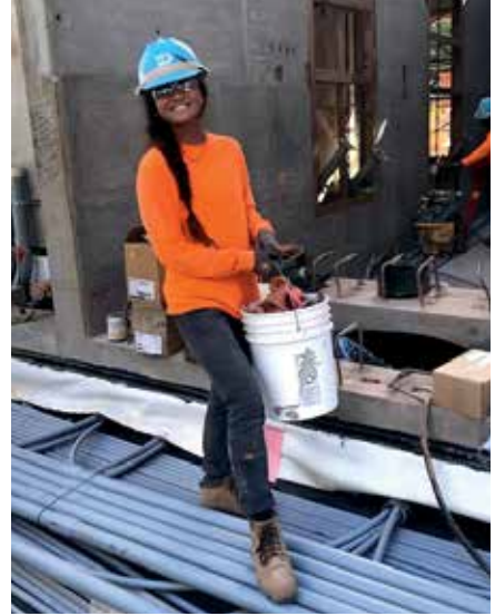
Erica Lee, carpenter apprentice, working on Hawaiian Dredging's Central Ala Moana project. PHOTO COURTESY HAWAIIAN DREDGING CONSTRUCTION CO.
