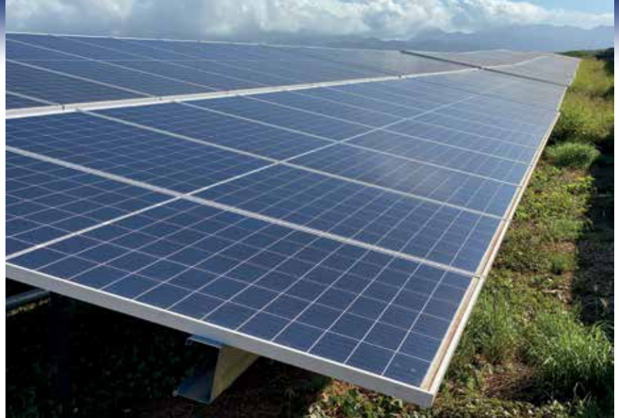
Hawaiian Electric's 20-megawatt West Loch solar project went on line last year.
