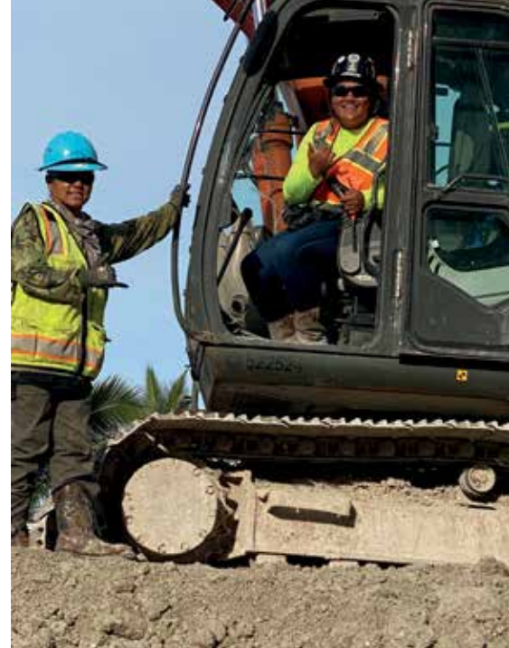
Jayar Construction Operating Engineers Florence Makinano and Pomaikalani Grube-Hose work on Hawaiian Dredging’s Koula project. PHOTO COURTESY HAWAIIAN DREDGING CONSTRUCTION CO.
