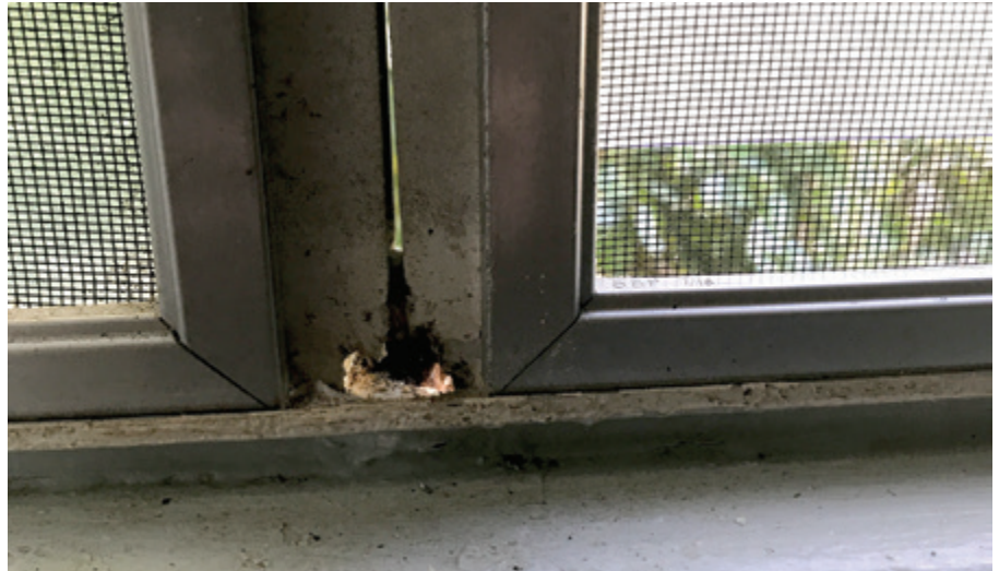
Corroded aluminum window frame
