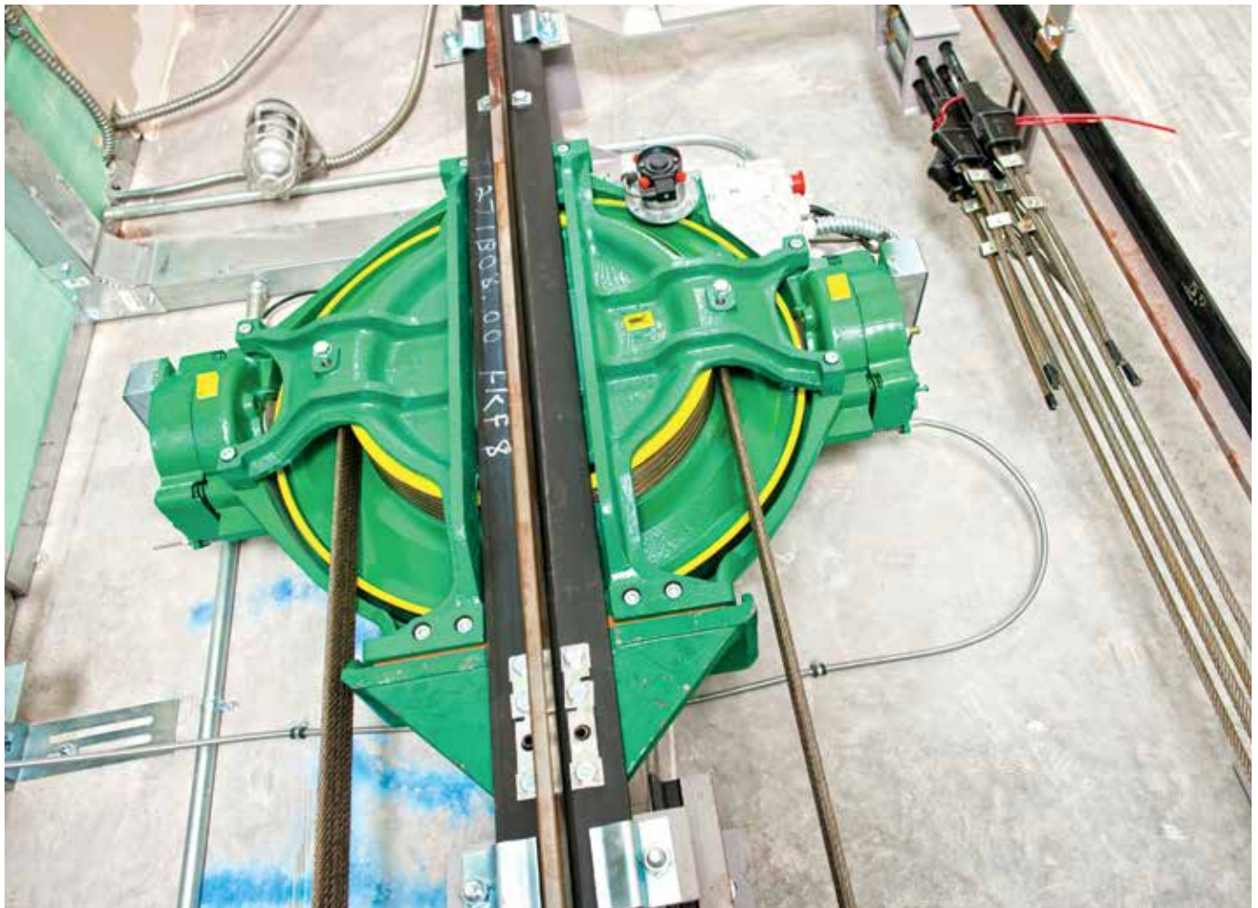
The KONE EcoDisk machine replaced six hydraulic elevators at Honolulu International Airport with an MRL (machine-room-less) traction elevator system.
