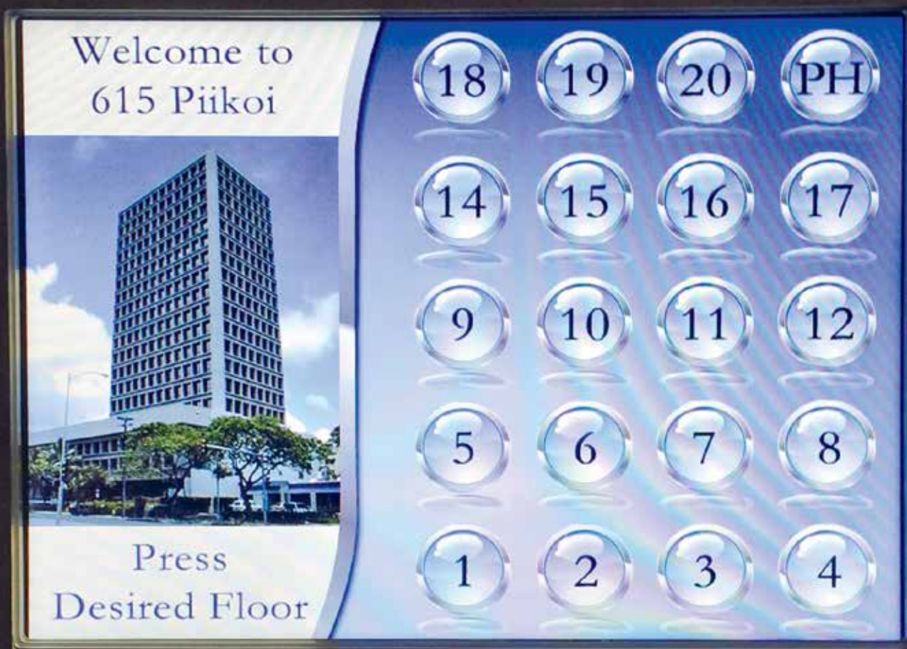
This touch-screen, destination dispatch kiosk directs people to an assigned elevator, cutting travel time.
