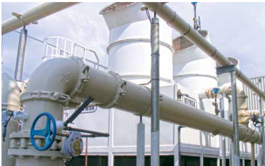
A water conditioning system must be kept clean from blockages caused by limescale.
