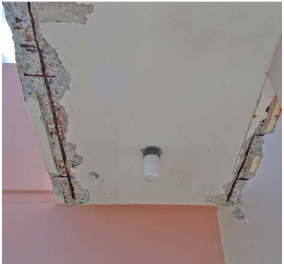
Without regular inspection and upkeep, spalling concrete can progress into an expensive repair job.
