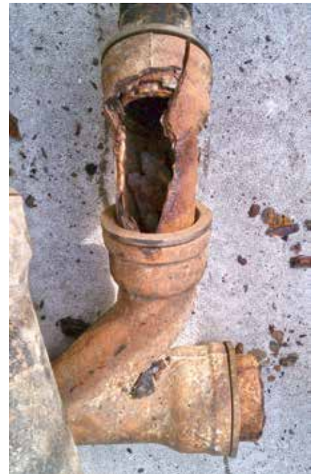
A small leak, if left unchecked, can quickly develop into a major problem.
