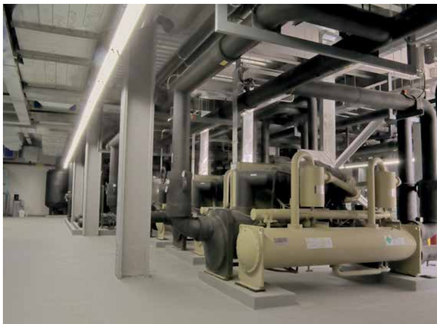
Tenants' comfort is the primary reason your chiller system should function at top capacity.
