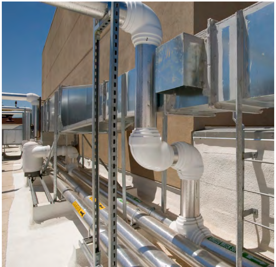
A periodic walk-through of the building helps the staff become familiar with its systems
