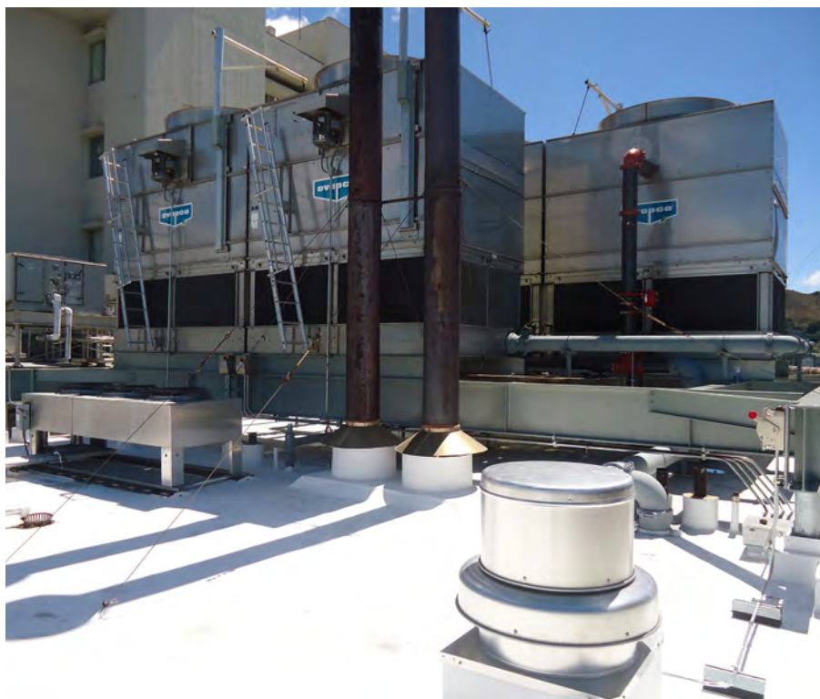
Financing agreements allow a property to install new equipment with minimal upfront costs
