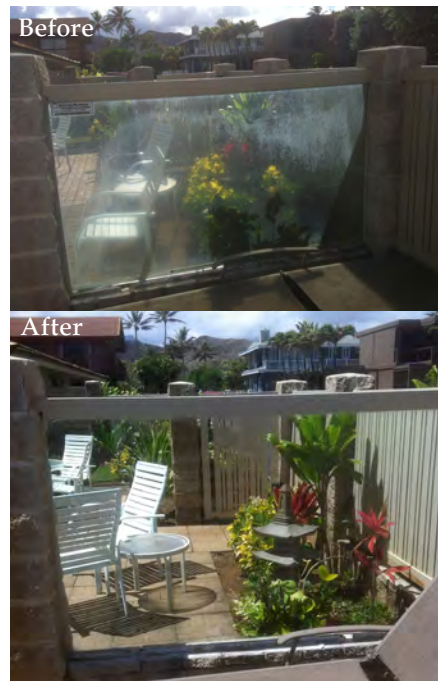
Hard water damage on glass, before and after treatment
